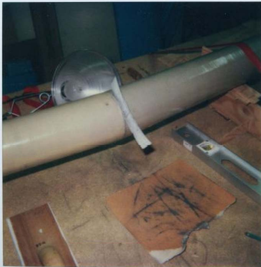
Butt joint of main spar sanded flush and verified with thin paper technique and spot-light technique 4/14/85
